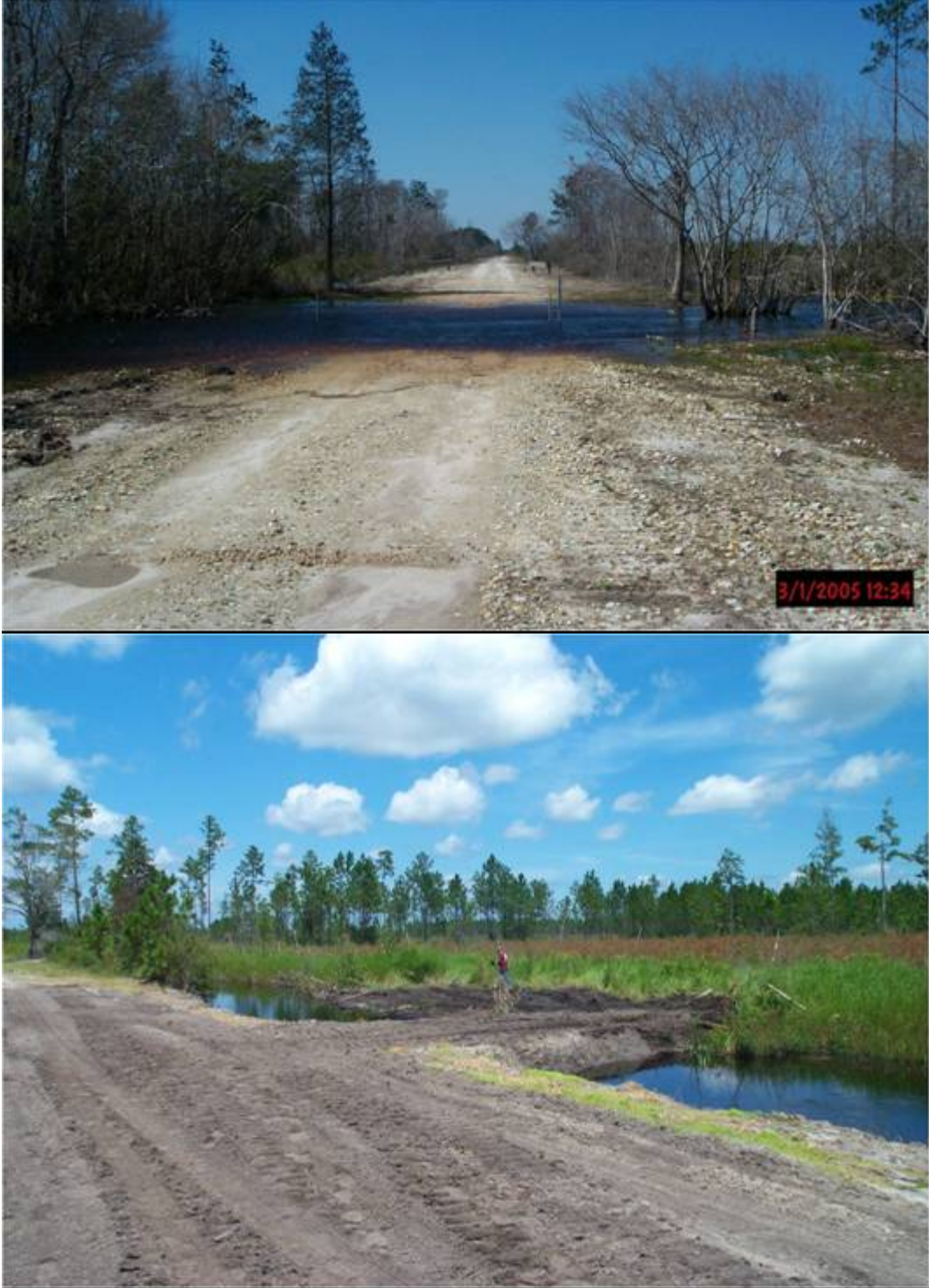
Figure 7. Typical views of hardened low-water crossing (upper panel) used to reconnect the historical flow way and ditch block (lower panel) used to redirect and retard flows
